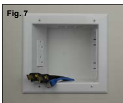
Figure 7: Your new Expandable Media Box with 20 Amp Duplex Receptacle is now installed and ready for the TV mount to be installed. Install your TV mount bracket per the TV bracket manufacturer's instructions.
