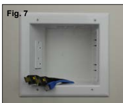
Figure 7: Your new Expandable Media Box with Duplex Receptacle is now installed and ready for the TV mount to be installed. Install your TV mount bracket per the TV bracket manufacturer's instructions.
